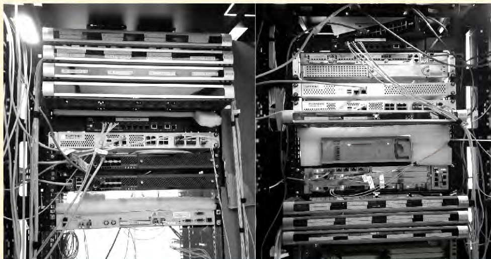
Redundant Firewalls (NGFW) at service
